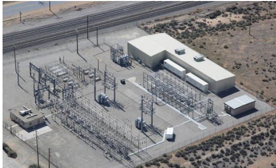
Tehachapi Energy Storage Project
