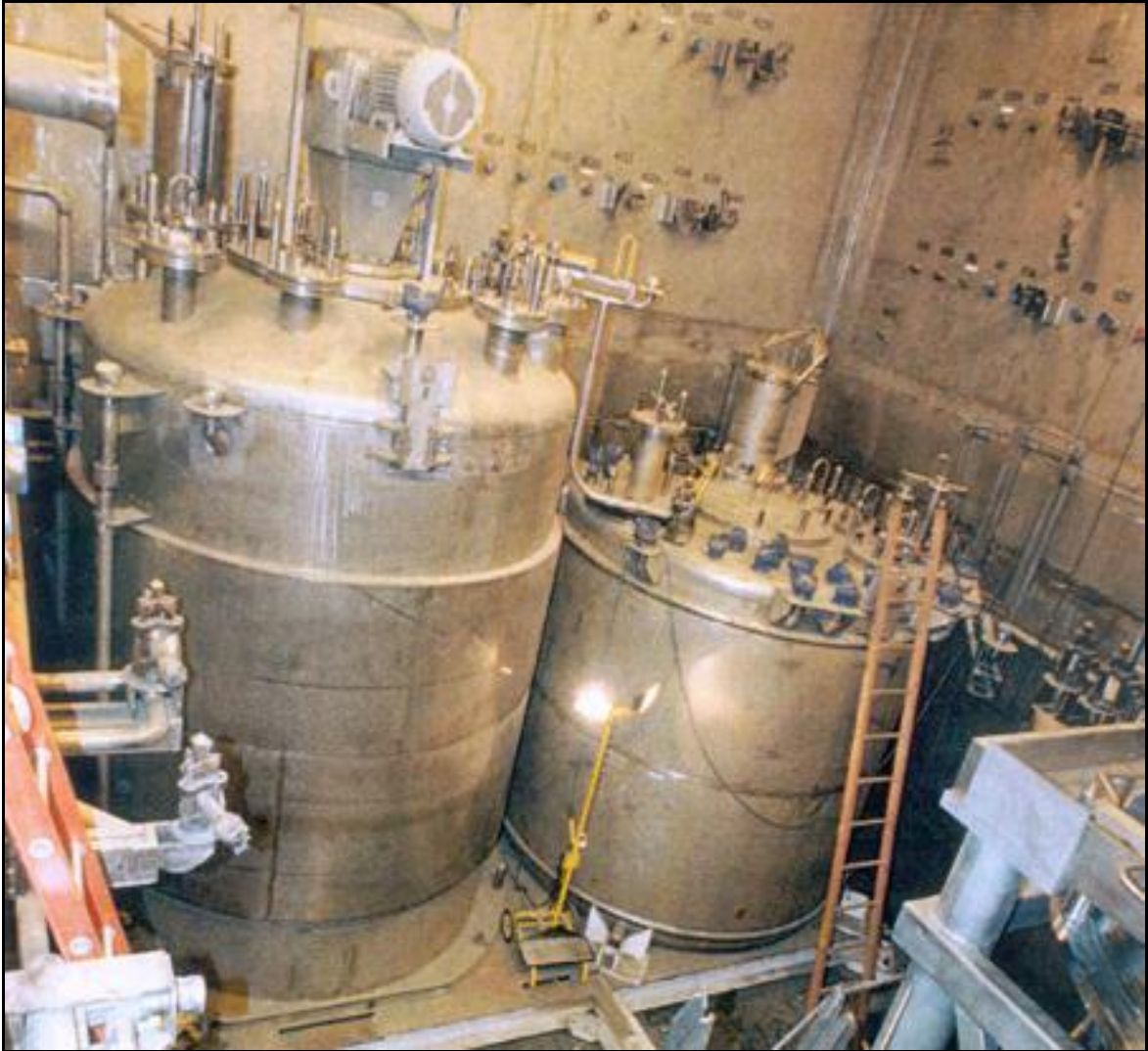
Figure 2-5. The Concentrator Feed Makeup Tank (left) and the Melter Feed Hold Tank Installed in the Vitrification Cell (WVDP photo)
