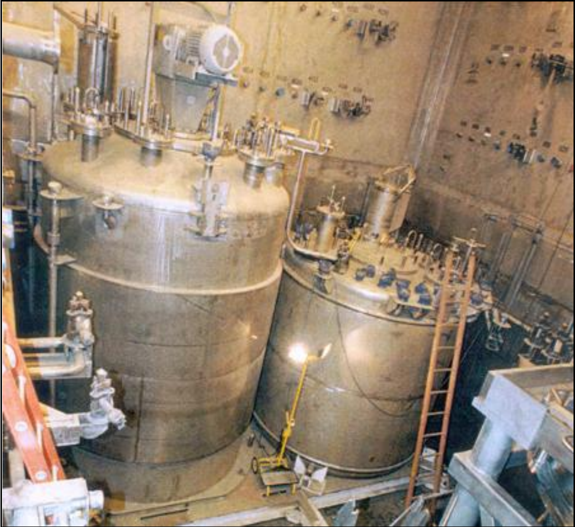
Figure 2-5. The Concentrator Feed Makeup Tank (left) and the Melter Feed Hold Tank Installed in the Vitrification Cell (WVDP photo)
