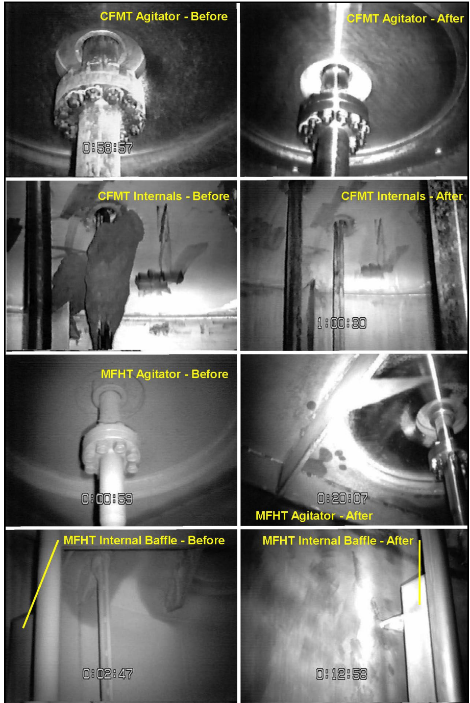
Figure 4-2. Before and After Flushing Images of the Two Vessels. (The shiny surfaces in the after images illustrate the effectiveness of the high-pressure washing in these WVDP photos taken with the underwater camera.) (from WVNSCO 2002f)
