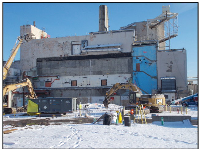
Completion of demolition of the Main Plant Process Building (MPPB) offices and Chemical Viewing Aisle (CVA)
