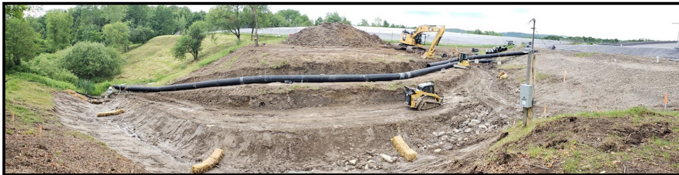
Construction of drainage improvements and erosion controls on the NDA north slope
