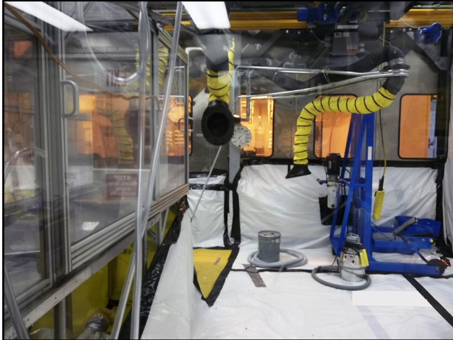
Container Sorting and Packaging Facility (CSPF)
