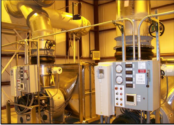
Two Replacement Ventilation Units (RVUs) for the MPPB exhaust through a single stack
