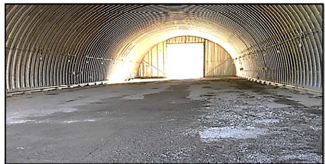
Chemical Process Cell - Waste Storage Area (CPC-WSA) emptied and prepared for closure
