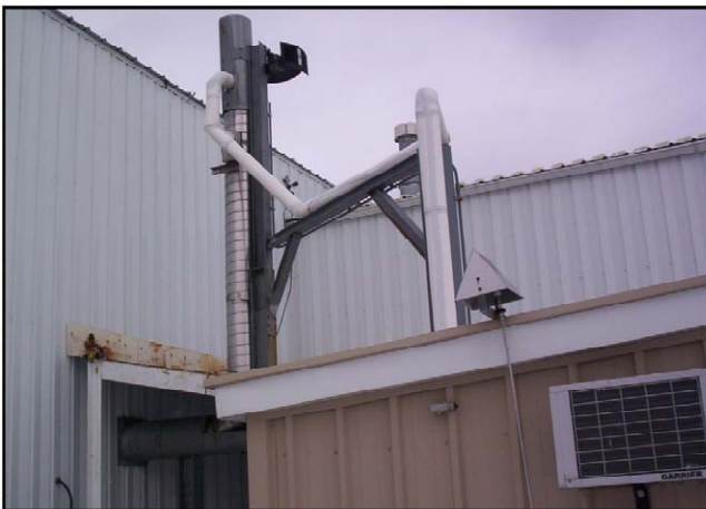
Container Sorting and Packaging Facility (CSPF) stack
