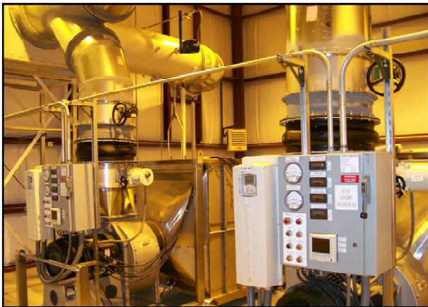
Two Replacement Ventilation Units (RVUs) for the MPPB exhaust through a single stack
