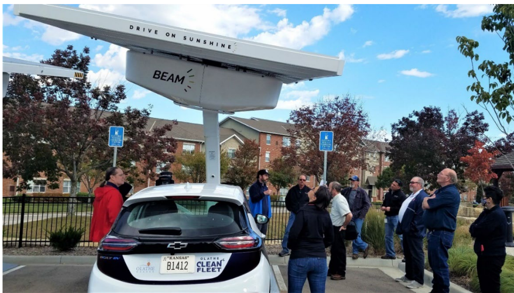
Figure I.4-2. The City of Olathe KS new EV and EVSE. (Photo credit: Jeff Windsor)
