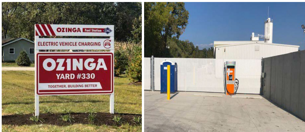
Figure I.1-1. EV charging station installed and commissioned by Ozinga Energy at New Buffalo, Michigan
