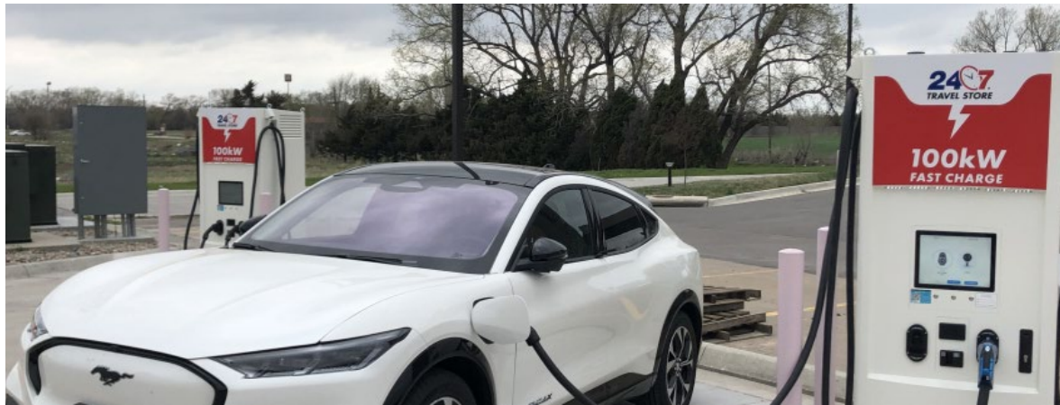
Figure I.4-1. The 24-7 Travel Store in McPherson, Kansas installed DCFC (Photo Credit: Tami Alexander)
