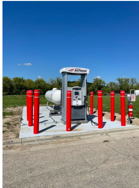
Figure I.1-4. ALCIVIA propane fueling station
