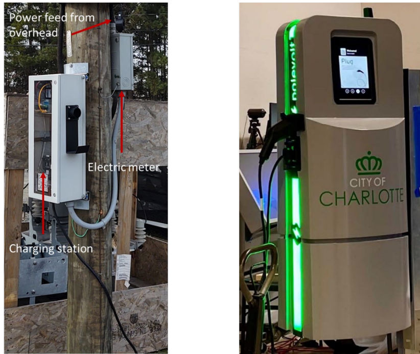
Figure I.11-3. Evolution of the charging station. Left: Initial prototype mounted on an overhead distribution pole at a test facility. Right: First commercial prototype.
