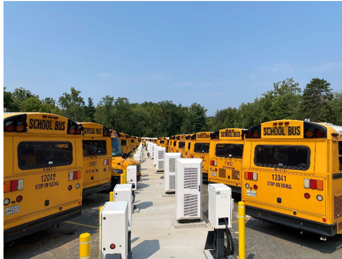
Figure I.31-2. Electric school bus chargers in the ground at the Bethesda, MD school bus depot where the first of the Montgomery County electric school buses will be deployed. Photo courtesy of Highland Electric.
