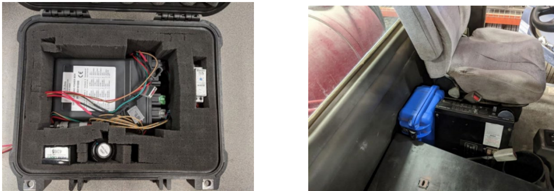
Figure I.17-1. HEM data acquisition system in Pelican case (left) and mounted in truck (right)
