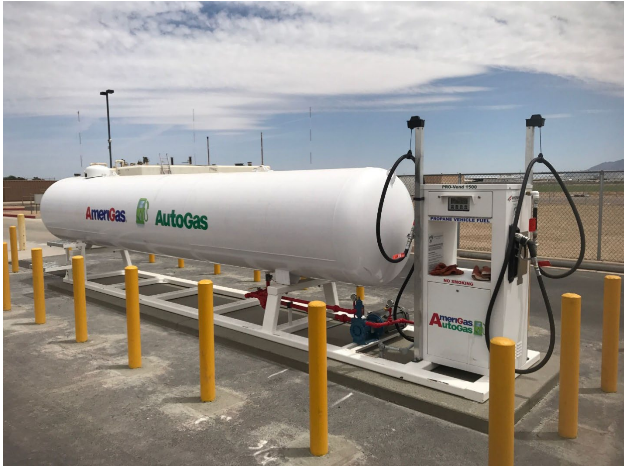
Figure I.36-2. Propane Autogas refueling infrastructure by AmeriGas and Superior Energy Systems, similar to propane fueling infrastructure to be provided by AmeriGas at Hi Pro, Inc. site. Photo credit: Superior Energy Systems
