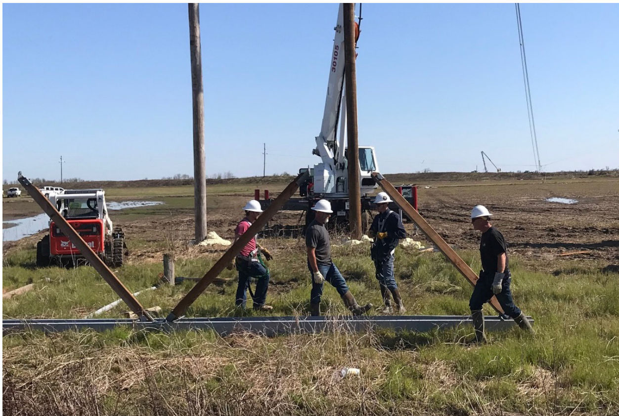
Construction crews were part of the team effort to install new structures following the storm.
