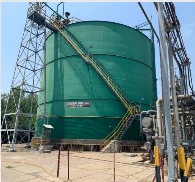
Ammonia Storage Tank at NFL, Nangal
