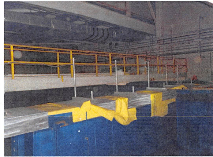
Fuel Receiving & Storage Area
