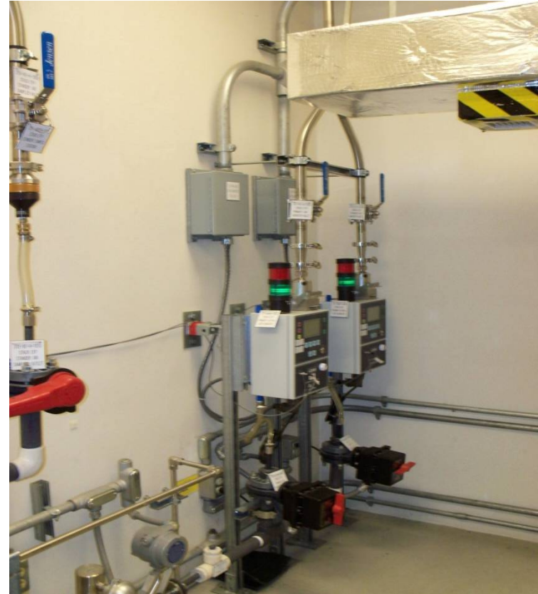
RHWF Stack Monitoring System
