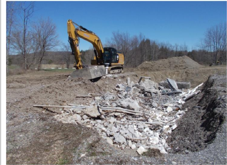
Completed the demolition of onsite equalization tanks, and began loading debris into intermodals
