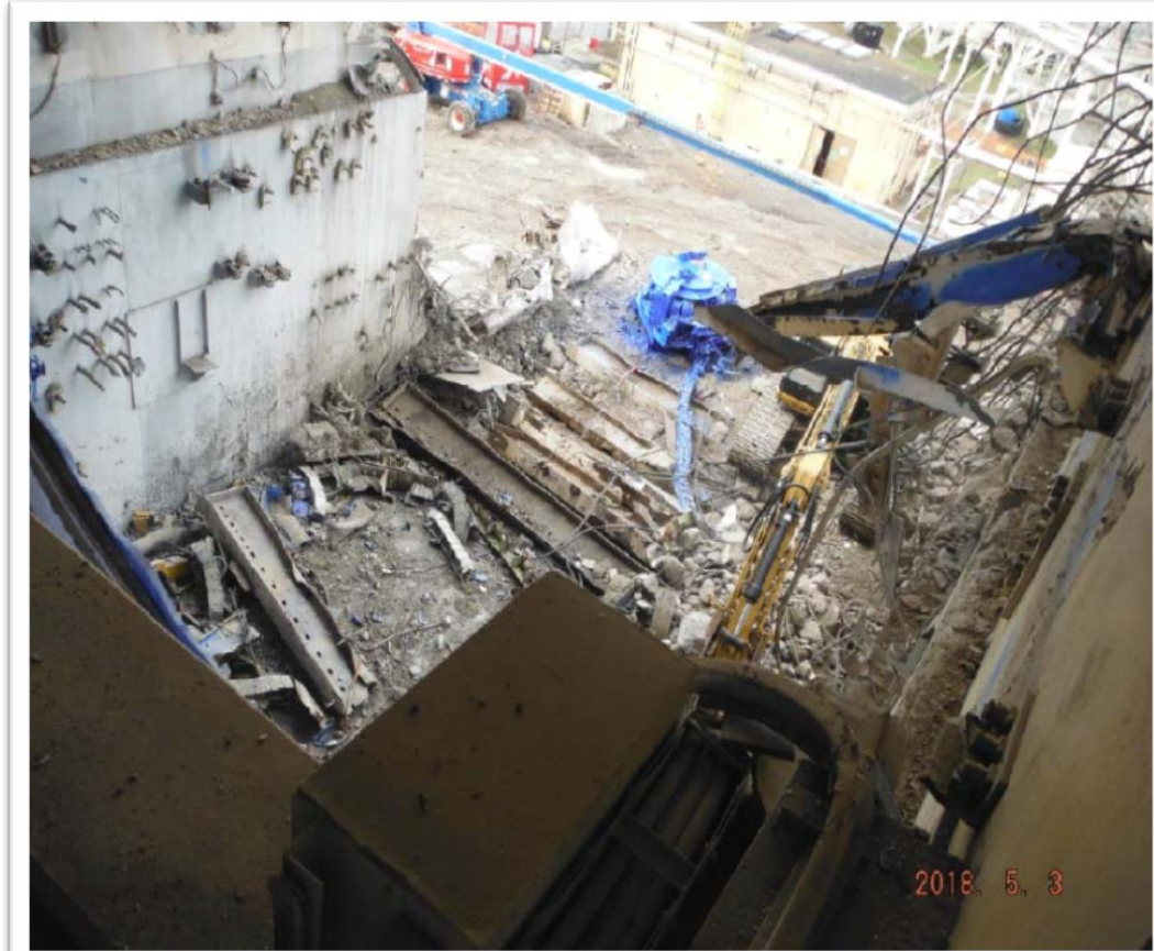
Vitrification process crane on floor May 3, 2018 (View from inside Vitrification Facility looking down )
