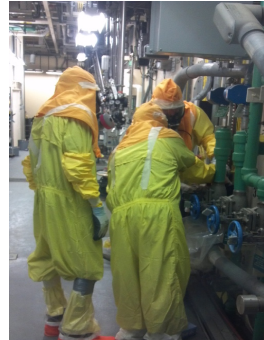
Out of Service Piping Air Gapping
