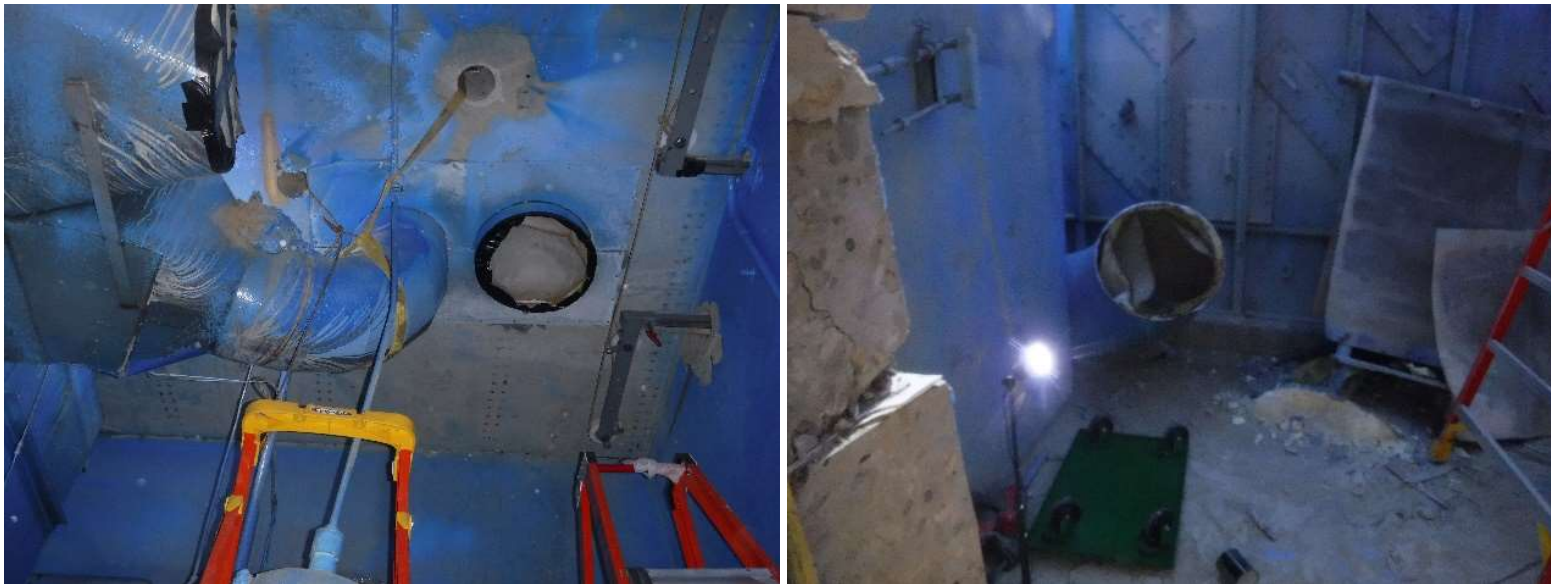
View of the vent duct to be cut by diamond wire saw (top) and duct after being cut (bottom)
