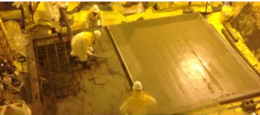
Filled EDR Soaking Pit
