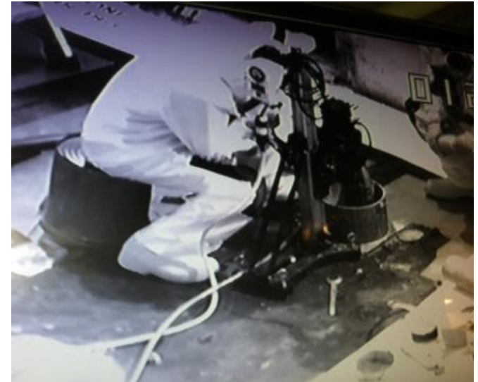
Core Boring in the Equipment Decontamination Room (EDR) – Added Floor Structural Enhancement
