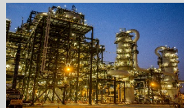
Natural gas processing
