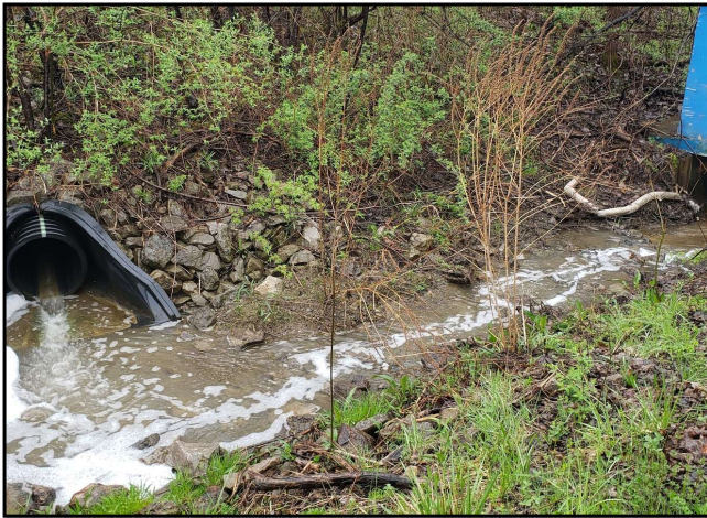
Culvert flowing into surface water sampling location WNSW74A on a tributary of Quarry Creek (See map location on Figure 2-3 )
