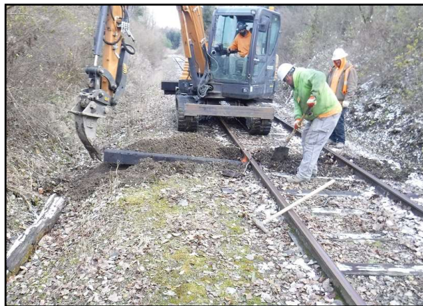
Maintenance work on rail line to ensure it is safe for use
