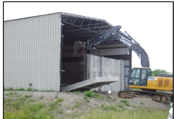
Renovations in progress for future use of the drum cell during MPPB demolition
