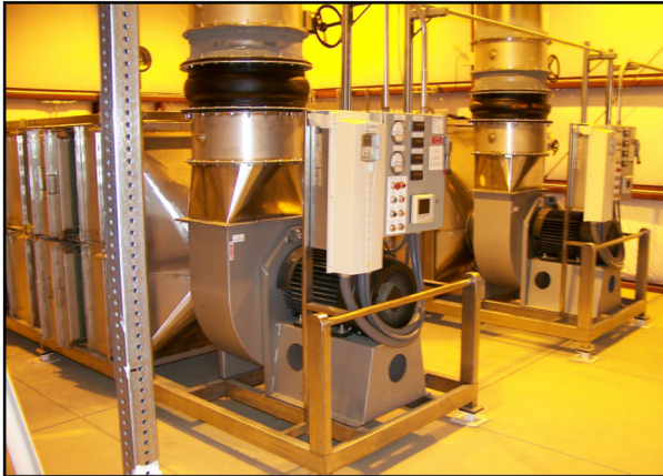
Replacement Ventilation for the MPPB (discontinued in early 2021)
