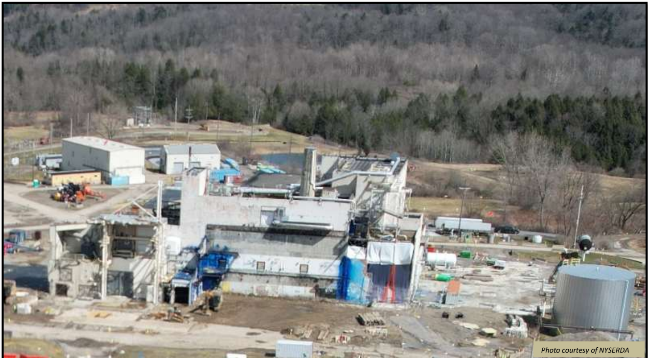
All ancillary structures demolished in preparation for Main Plant Process Building (MPPB) demolition
