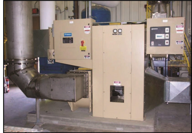
Ventilation of underground HLW tanks by the Tank and Vault Drying System (T&VDS)
