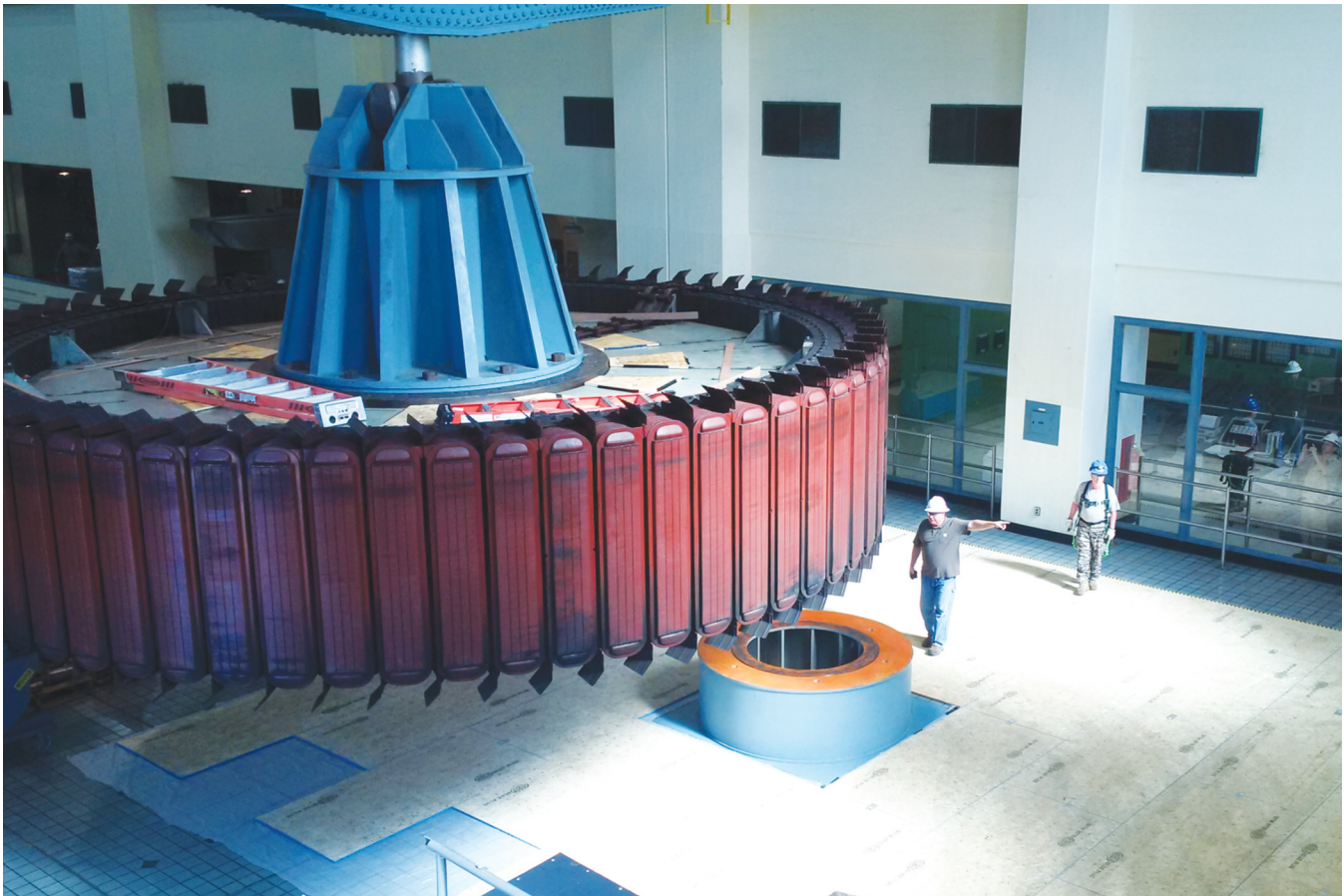
One of Center Hill's generator rotors is being guided to the rotor pedestal. There is only one location in the plant, other than the operating position from whence it came, structurally designed to support the weight of the heaviest of rotating generator components. Center Hill's fully assembled rotors weigh in at a modest 242 tons.
