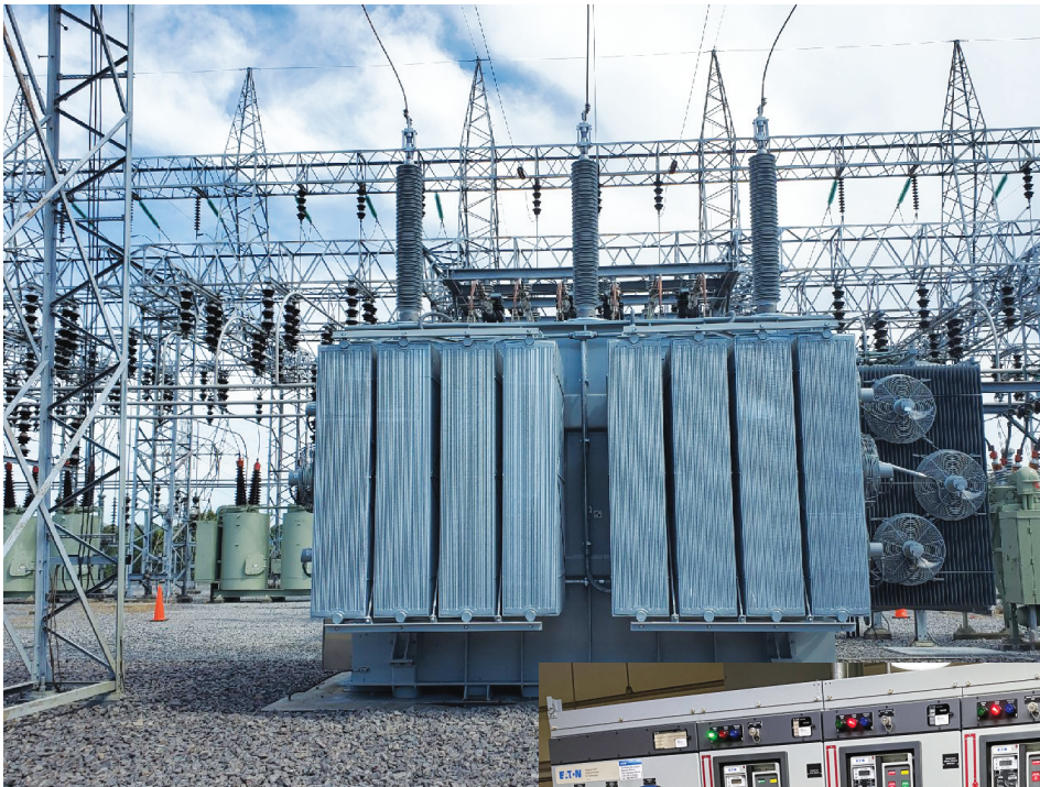
A new transformer, which steps up the generator voltage to transmission voltage, is installed in the Barkley switchyard.
