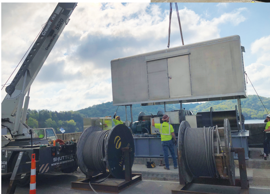
A generator intake gate lifting mechanism is being replaced at Center Hill. These devices were also replaced at Dale Hollow and Wolf Creek.
