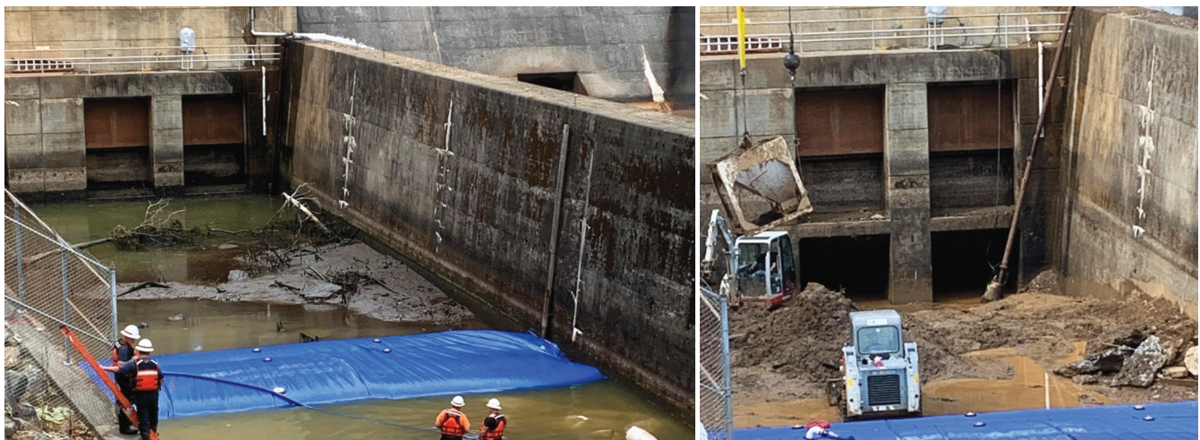
Landslide cleanup continued through 2021 at Philpott. In these photos, the powerhouse tailrace is unwatered to remove debris and excavate mud from the generator draft tubes (square openings lower right). The draft tube is the final water passage through the dam below the generator turbines.
