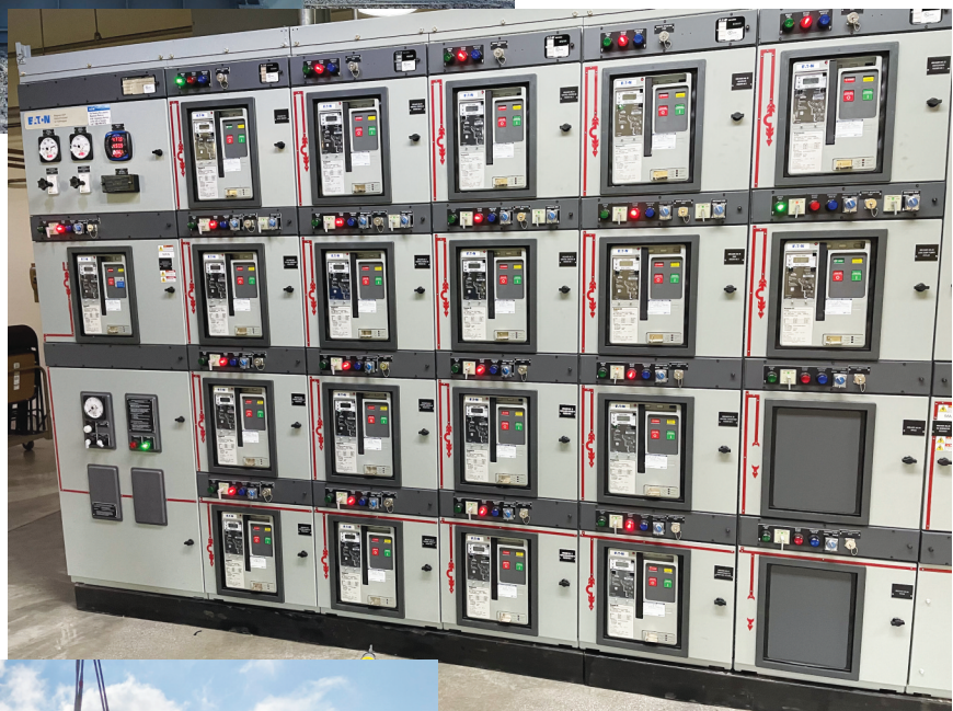
New arc flash maintenance personnel safety compliant station service switchgear breakers are installed at Wolf Creek to distribute power throughout the facility.
