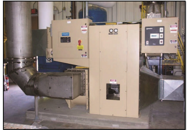
The Tank and Vault Drying System (T&VDS) exhausts through the Supernatant Treatment System (STS) stack
