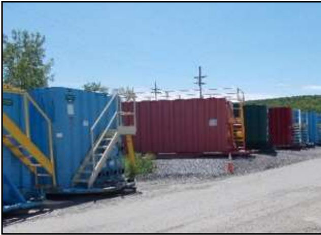
Storage tanks for the new water management system to support MPPB demolition
