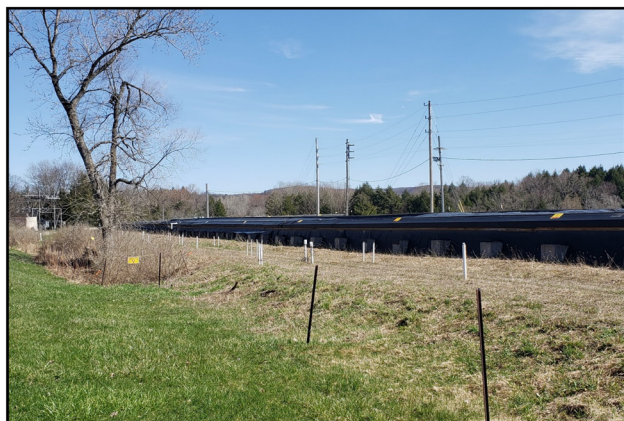
Permeable Treatment Wall (PTW) (below ground) and soil removed (black covered structure in background)
