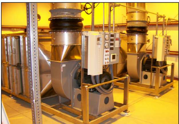
Replacement Ventilation System (RVS)
