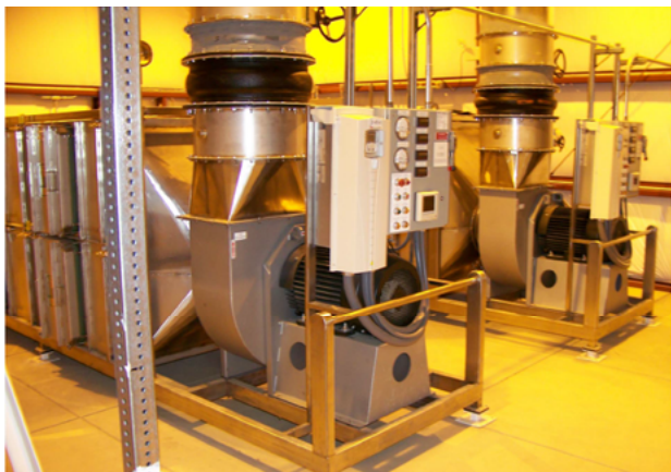
Replacement Ventilation System (RVS) for a portion of the MPPB
