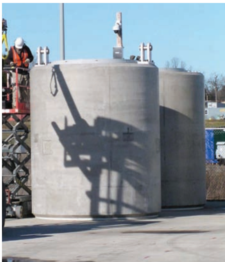
Four casks were placed on the interim HLW Cask Storage Pad in 2015
