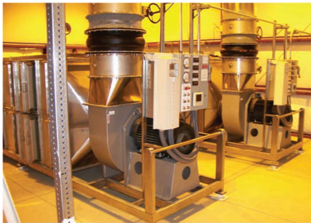
MPPB HEV Replacement Ventilation System (RVS)
