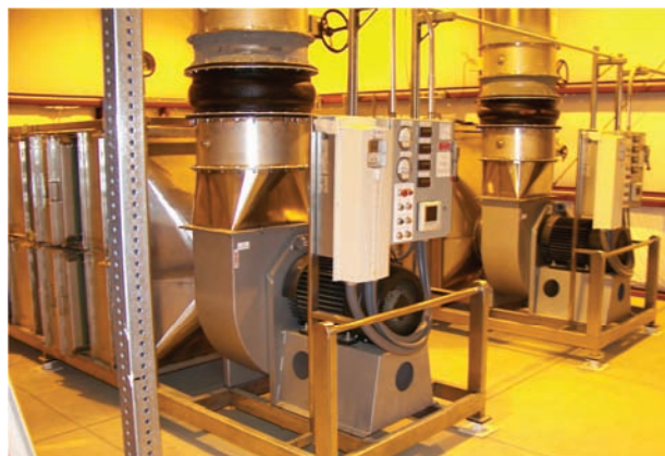
MPPB HEV Replacement Ventilation System (RVS)
