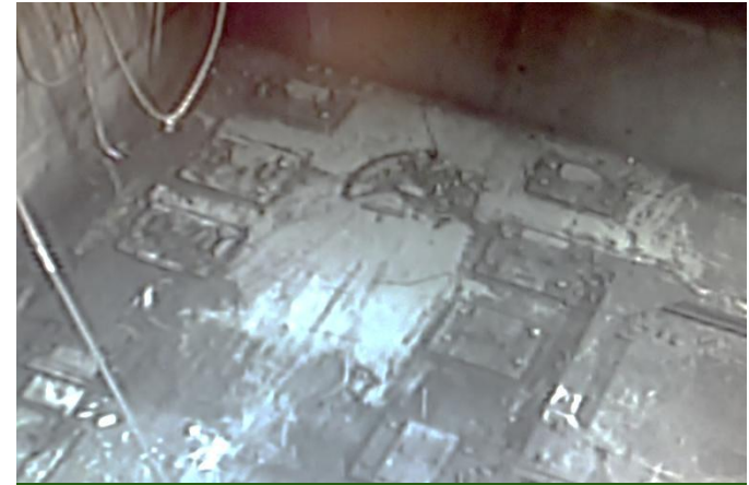
Vit Cell Equipment Pit after Vacuuming
