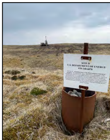
The team used a drill rig at Site D to assist with repairs.
