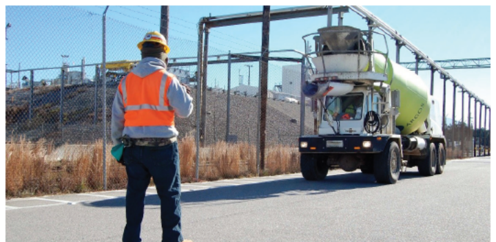
The final operational closure activity begins with workers pouring specially formulated grout (a cement-like substance) into the approximately one million-gallon capacity tank.
