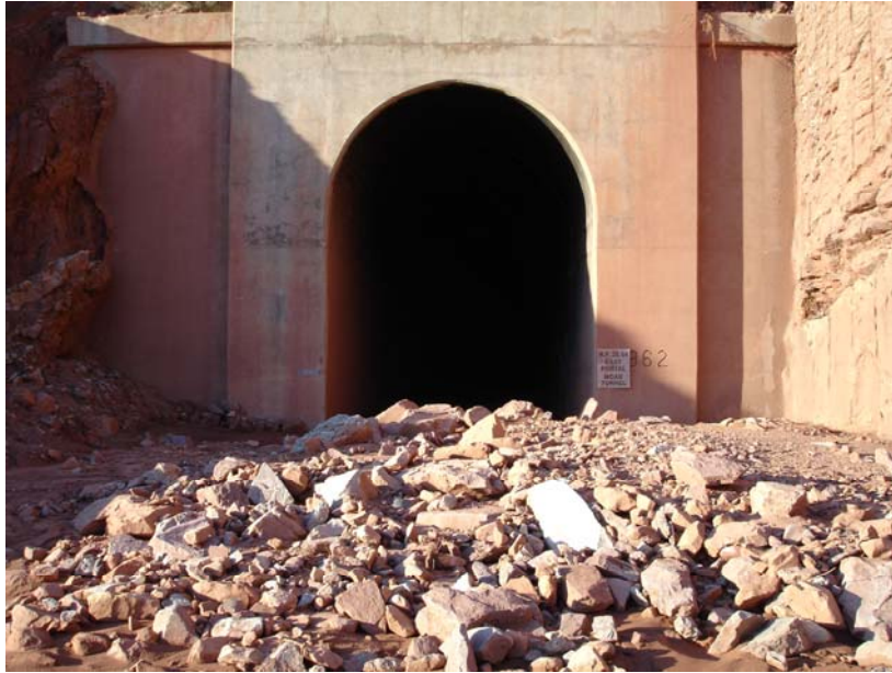
Photo 24. Rockfall Near Portal
