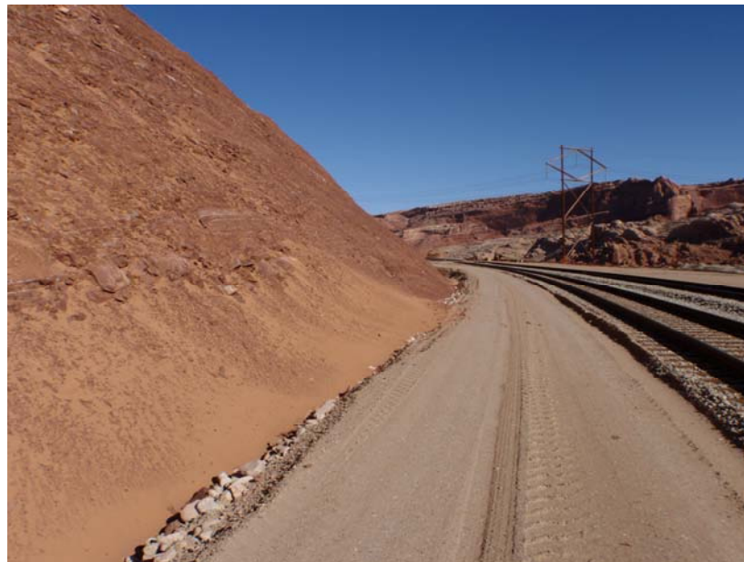
Photo 29. Windblown Sand in Drainage Ditch Along New Moenkopi Exposure on Excavated Hillside
