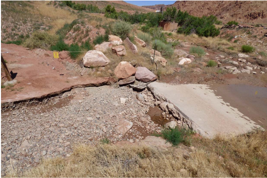
Photo B-23. Moab Wash Lower Crossing Erosion Damage
