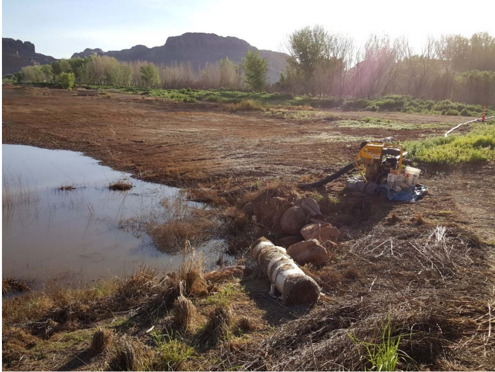
Photo C-1. Trash Pump Set Up at Southern End of Well Field
