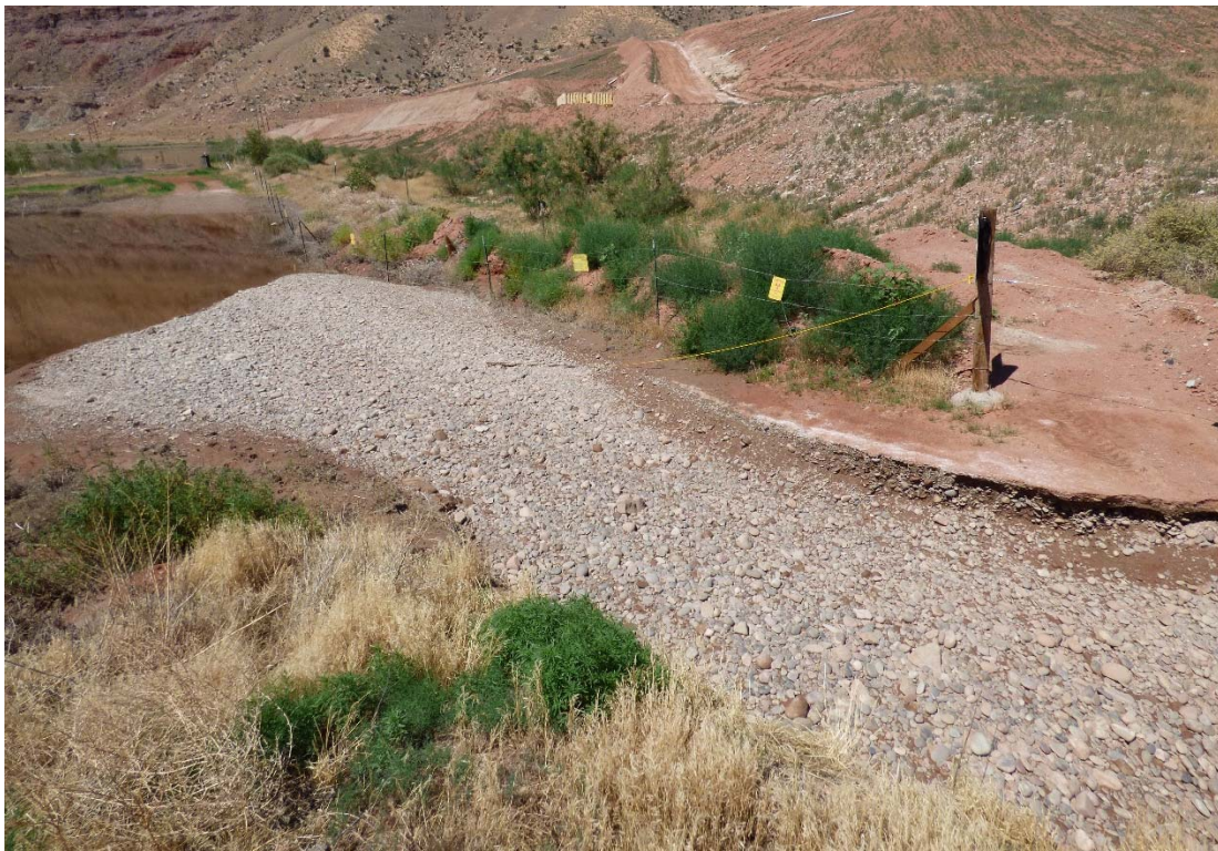
Photo B-24. Moab Wash Lower Crossing Exposed Gravel
