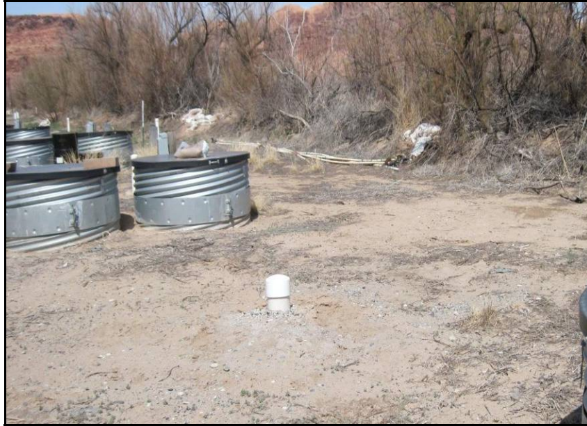
CF2 Remediation Well 0651
