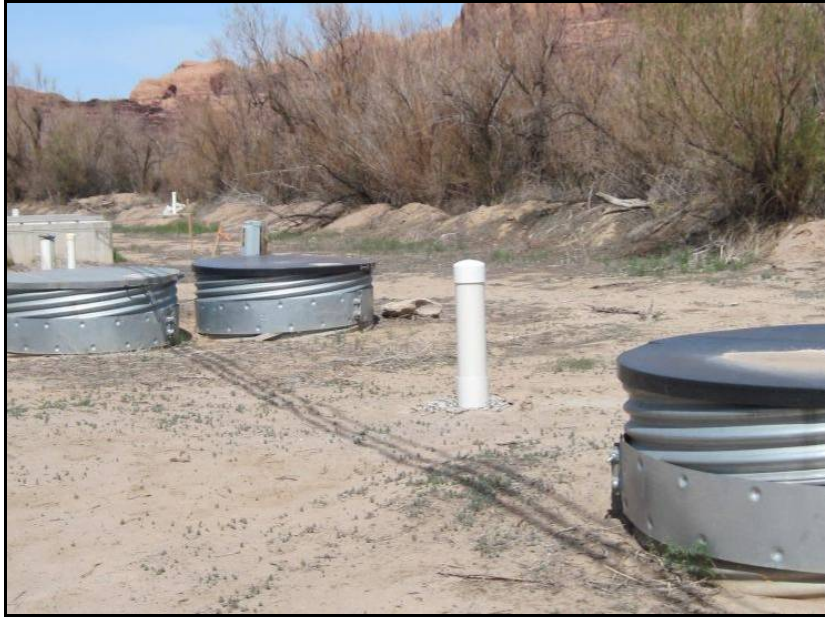
CF2 Remediation Well 0653
