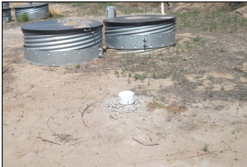
CF2 Remediation Well 0652
