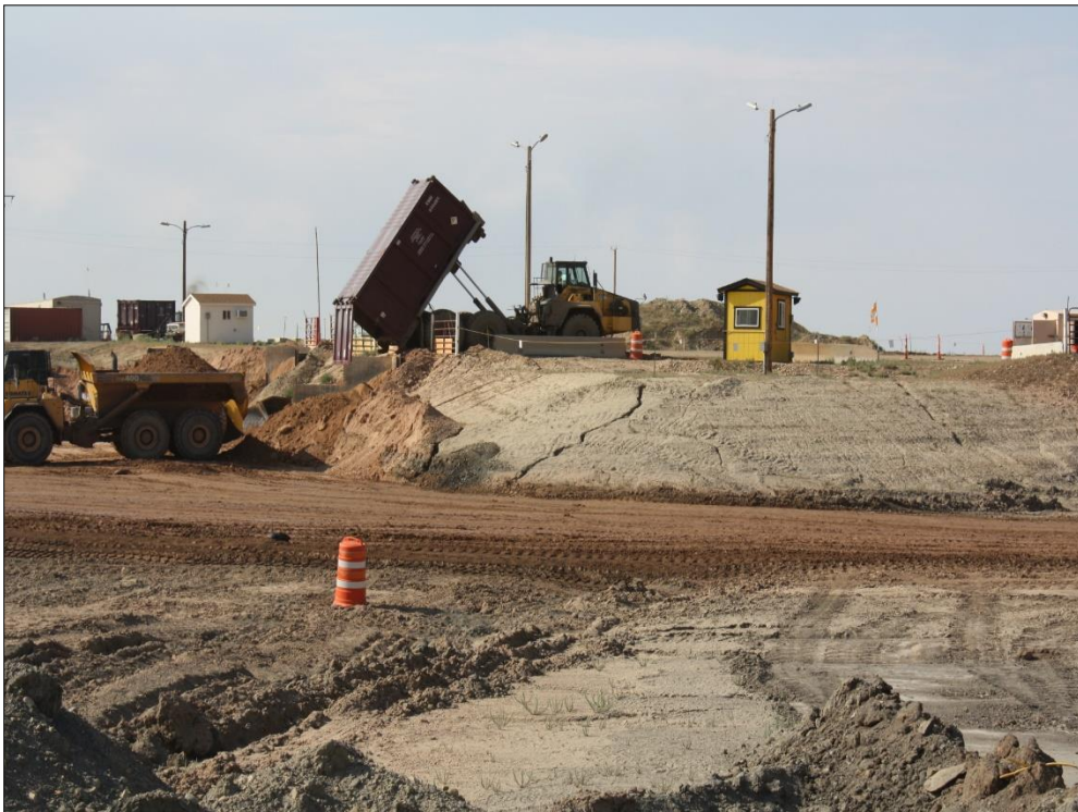
Photo 24. Container Dumping August 29, 2017
