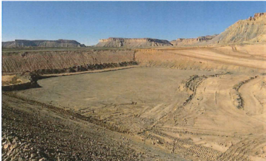
Photo 4 Cell Floor Following Dump Ramp Removal (note: edges of the ramp remain)
