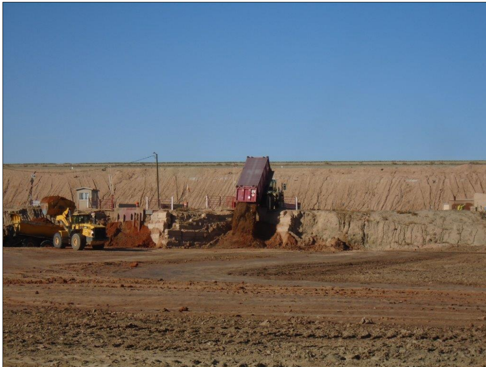
Photo 8. Modified Container Dumping November 6, 2014
