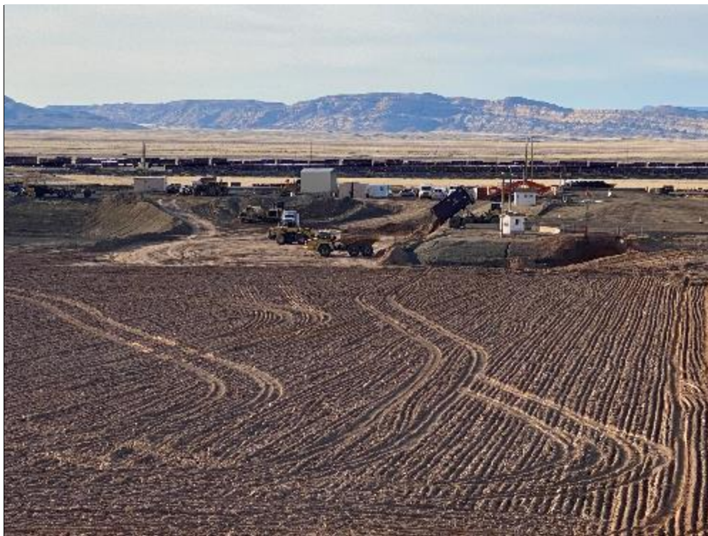
Photo 40. RRM Lifts March 2021
