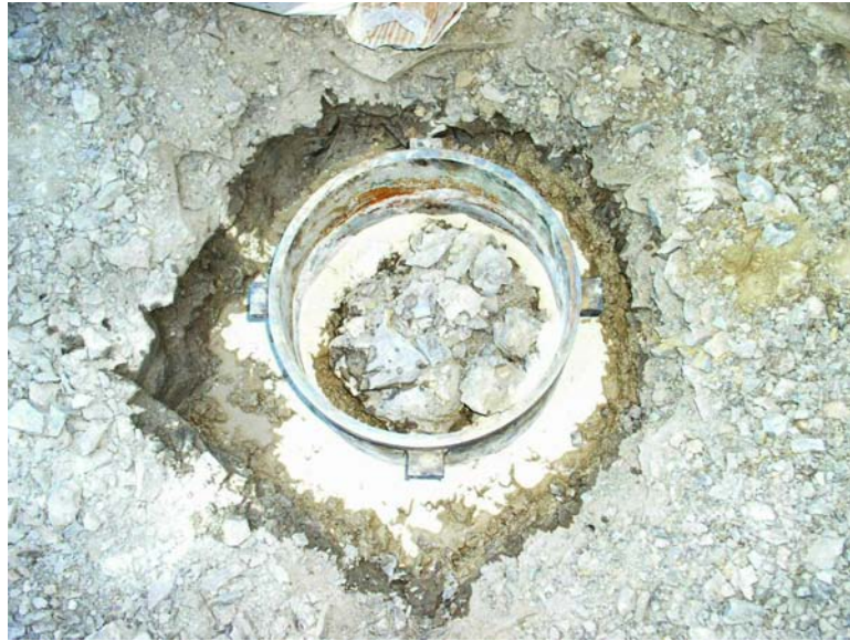
Figure 5. AEP Ring Placed in Channel With Bentonite Prior to Adding Water to Fully Hydrate Bentonite
