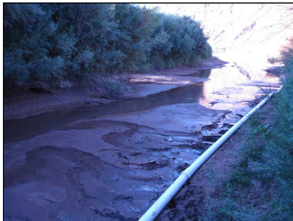
Photo D-20. CF4 Channel With Initial Action Piping (view to south)
