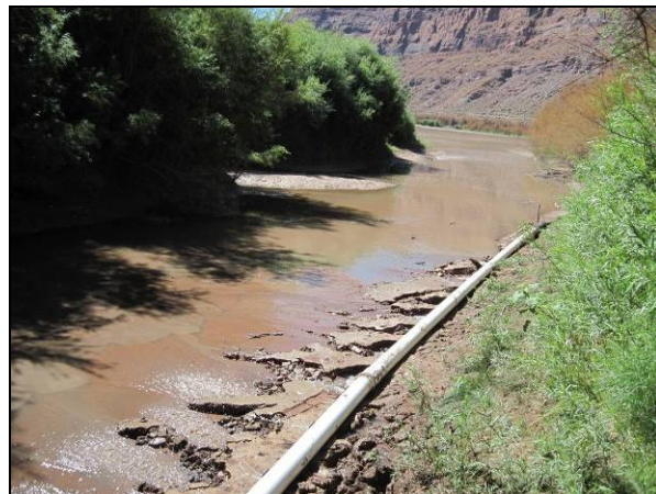
Photo D-17. CF4 Channel With Initial Action Piping (view to south)
