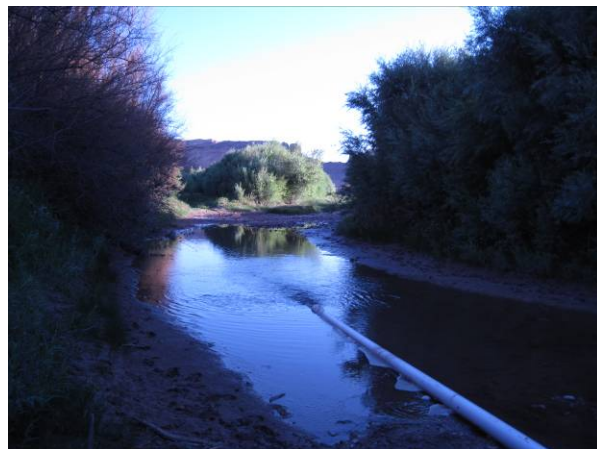
Photo D-19. CF4 Channel Towards Confluence With Initial Action Piping (view to north).
