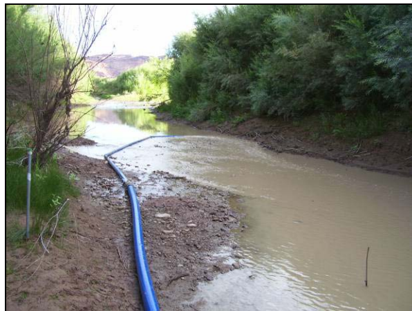
Photo 29. CF4 channel with initial action (view to northeast)
