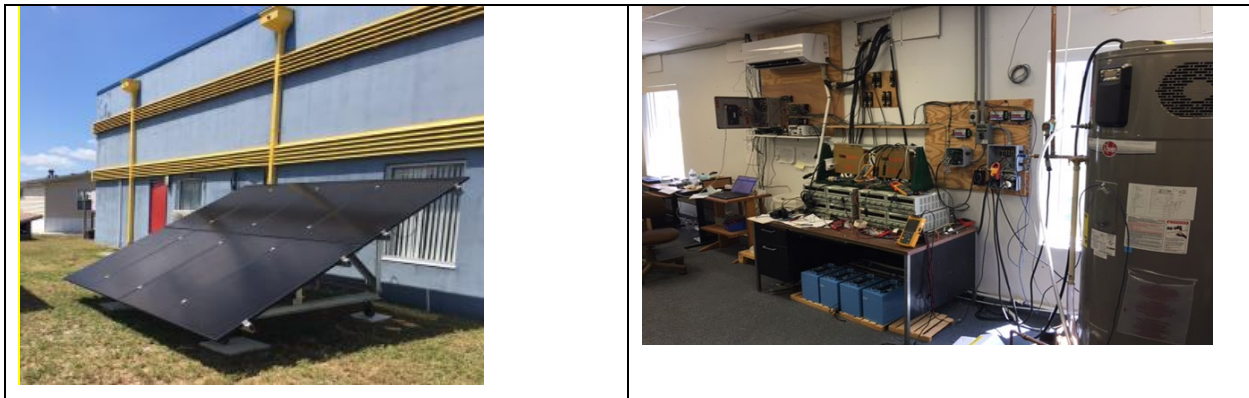
Figure C-2. Photos of System C components installed in the Building Science Lab.
