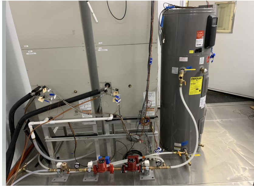
Hot water tank
