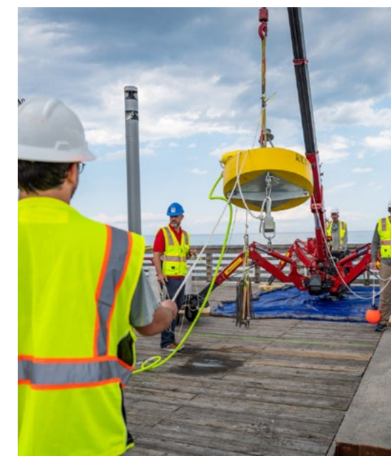
Team members deploy a preliminary testing device that supports foundational research for small, modular, wave-powered desalination systems at Jennette's Pier in Dare County, North Carolina. Photo by Coastal Studies Institute
