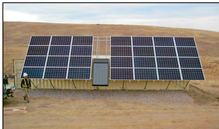
Solar installation at Rocky Flats Site, Colorado.
