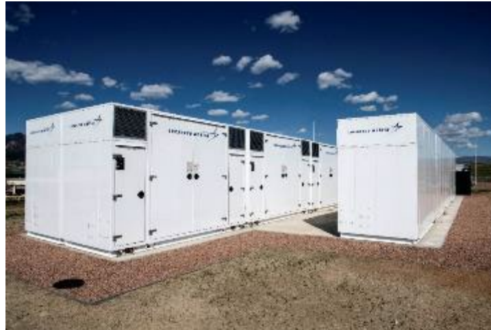
Fort Carson Battery Energy Storage (ESPC-funded)
