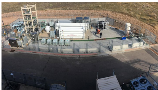
Figure 1. The new heavy-duty hydrogen station at the NREL Energy Systems and Integration Facility in Golden, Colorado.
