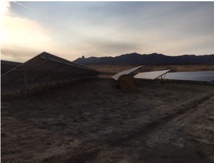
Sunset on Towaoc Community Solar Array, Left Toe Sleeping Ute Mountains Backdrop
