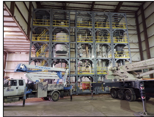
Autothermal pyrolysis demonstration plant (50 ton per day) near completion in Redfield, IA
