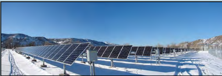
New solar array on the New Rifle, Colorado, Processing Site.
