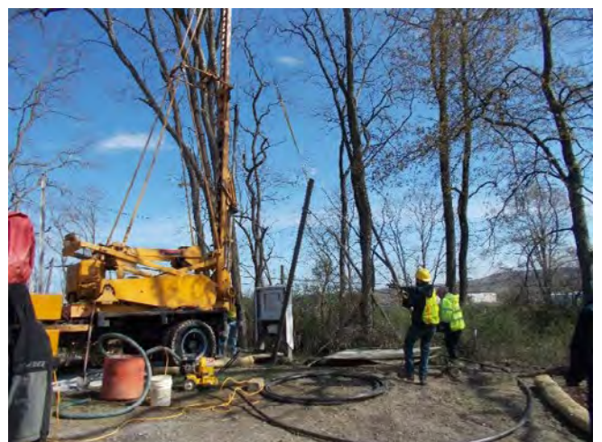
Workers remove the steel well casing from a former schoolhouse site and restored the area.
