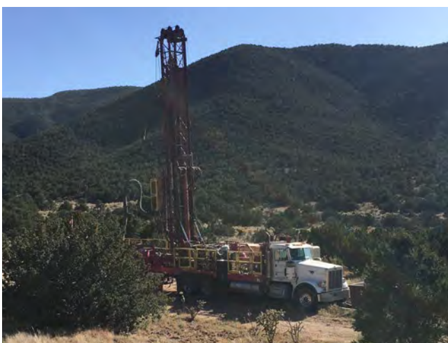
Installation of a groundwater monitoring well at the Burn Site Groundwater AOC.
