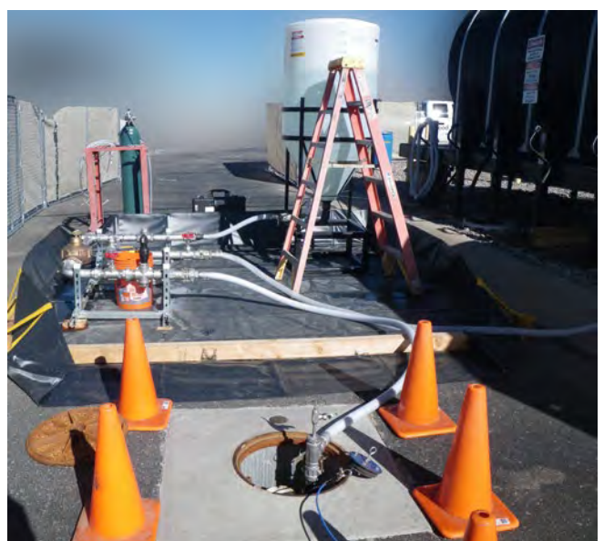
Injection of bioremediation agents into the groundwater for potential cleanup of contaminants during the TA-V Treatability Study.
