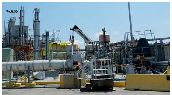
SRS completed modifications to convert Tank 42 into the third blend tank for the SWPF feed. Pictured is the site of Tank 42.
