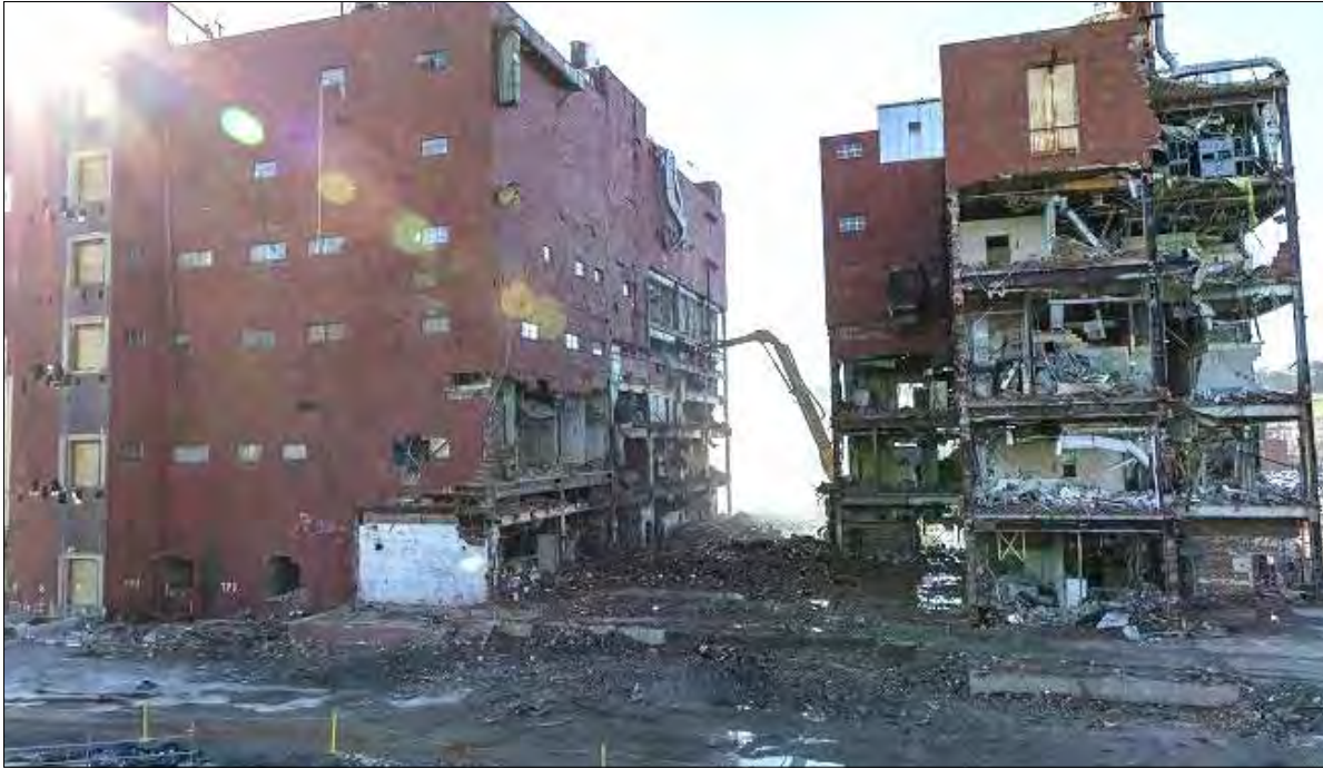
Demolition began on the last remaining facility in the Biology Complex at Oak Ridge in March. Building 9207 stood six stories tall and spanned 255,000 square feet. Tear-down of the final buildings — 9207 and 9210 — generated 118 million pounds of debris.
