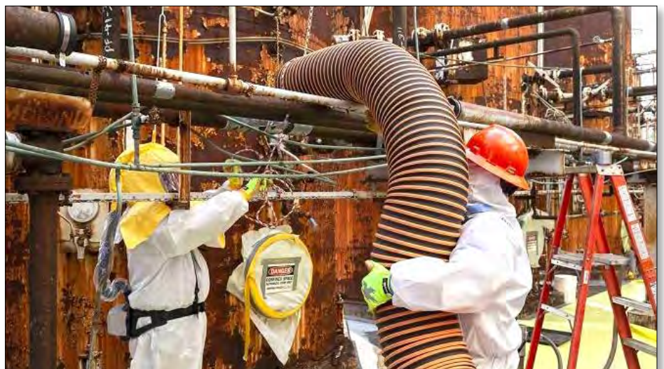
Oak Ridge workers remove mercury and mercury-contaminated solids from process pipes in the column exchange, or COLEX, equipment at the Alpha-4 facility at Y-12.
