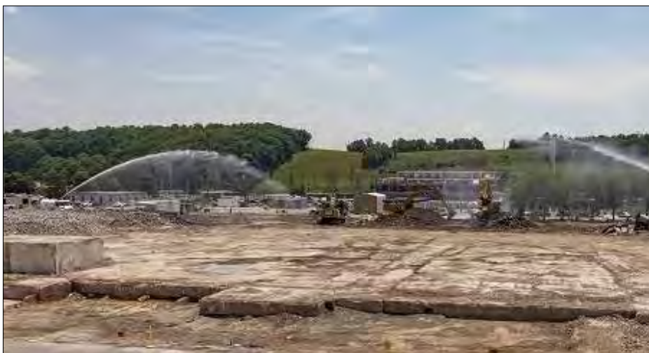
A view of the Biology Complex slab after demolition. Workers are actively removing the buildings’ foundations, which is slated for completion early next year.
