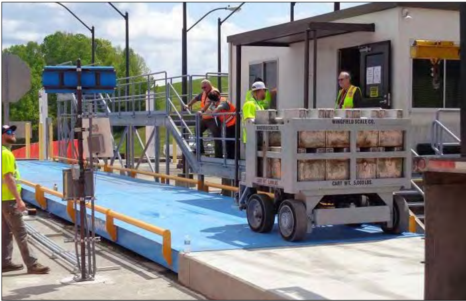
Crews installed a new truck scale at the Oak Ridge Reservation Landfill earlier this year as part of upgrades to waste management operations at Oak Ridge.
