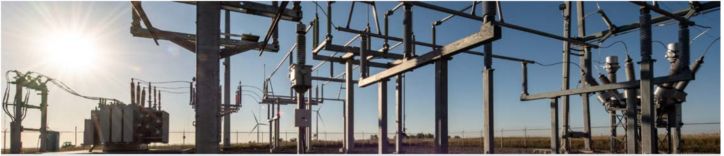
NREL's new 19.9-MW substation, used for ARIES utility-scale grid integration research. Photo by Dennis Schroeder, NREL
