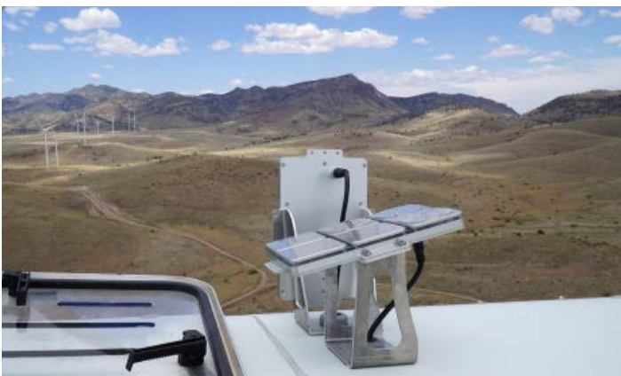
Two NRG devices mounted on top of a wind turbine nacelle, one pointing upward toward the blades, and one pointing to the right of the turbine. Photo by Harrison Gatos, NRG Systems
