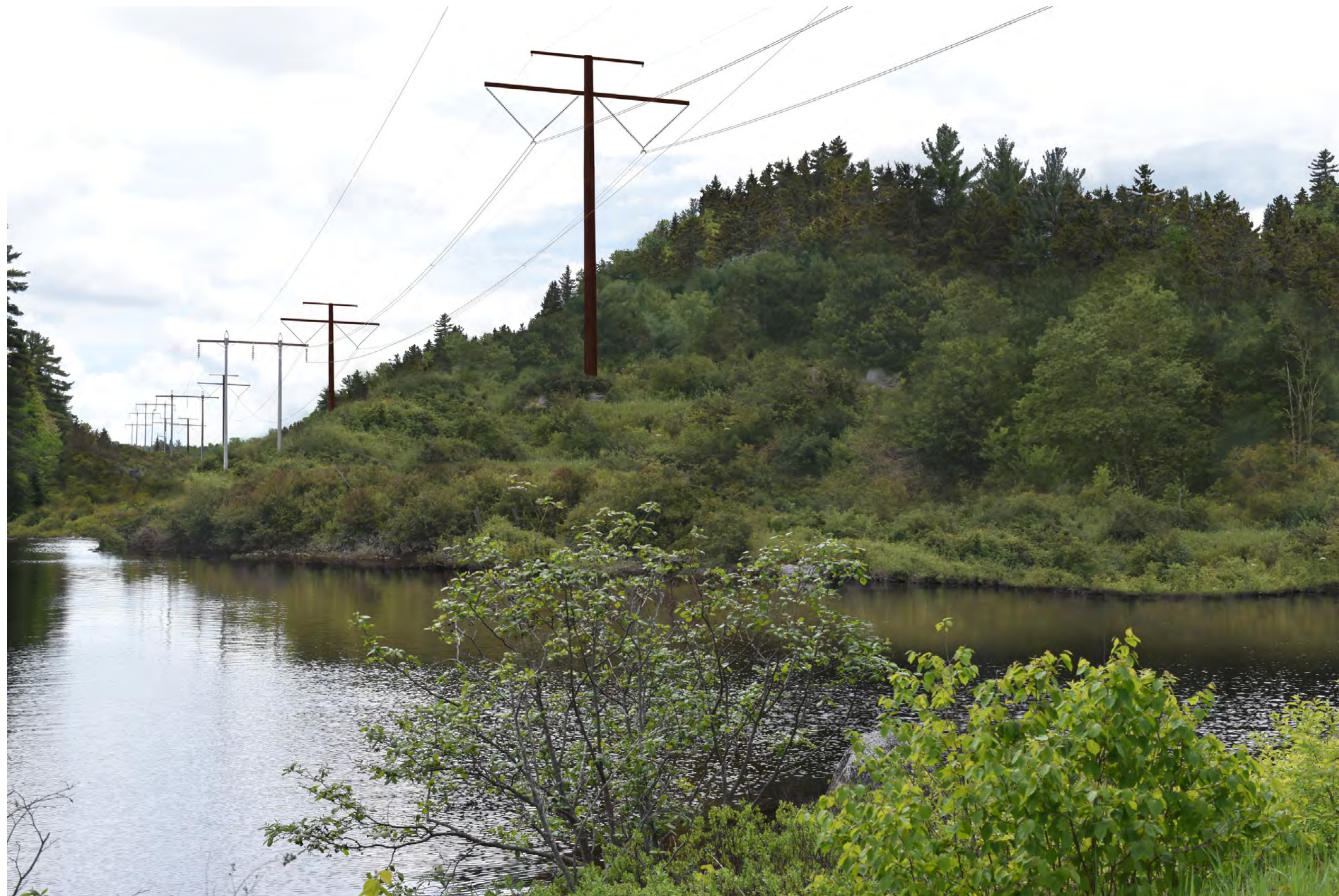
Proposed Conditions: Normal view looking south on Troutdale Road looking toward Joes Hole toward the proposed co-located HVDC transmission line. Over a distance of approximately 4,400' within the vicinity of the Appalachian Trail crossings, tapered vegetation management techniques will be used in both the existing 125' wide transmission line corridor and the proposed 75' widened corridor. Portions of six HVDC structures will be visible from this viewpoint. This photosimulation illustrates vegetation re-growth anticipated within 10 to 15 years after installation.
