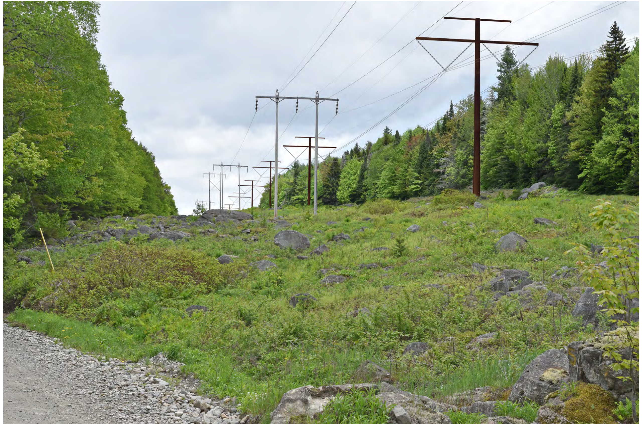
Photosimulation 18A: Normal view looking southeast from Troutdale Road toward the proposed co-located HVDC transmission line. The existing 150' wide corridor clearing will be widened by 75' on the western side to accommodate the new transmission line. Six HVDC transmission structures will be visible looking to the southeast.
