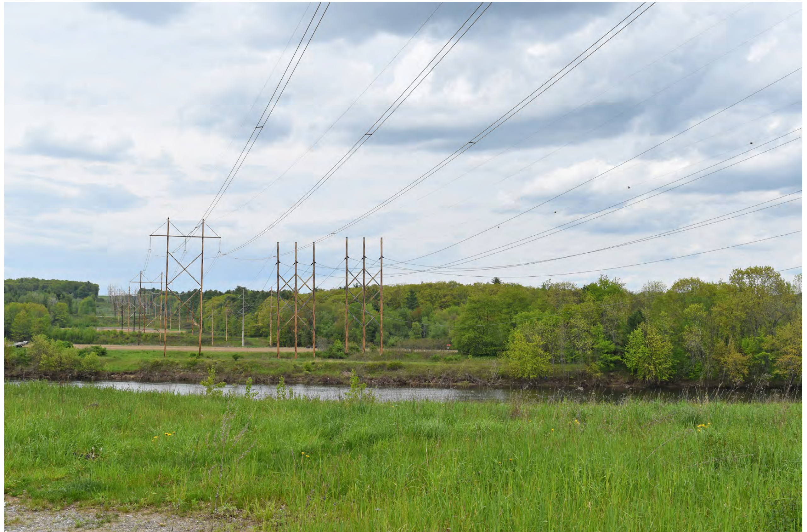
Photosimulation 25A: Normal view looking from northeast from Riverside Road / Route 136 toward the proposed Sections 62 & 64 Rebuild transmission line. The wood H-frame 115 kV structures will be replaced. No additional tree removal will be required. 20 +/- of structures will be visible.
